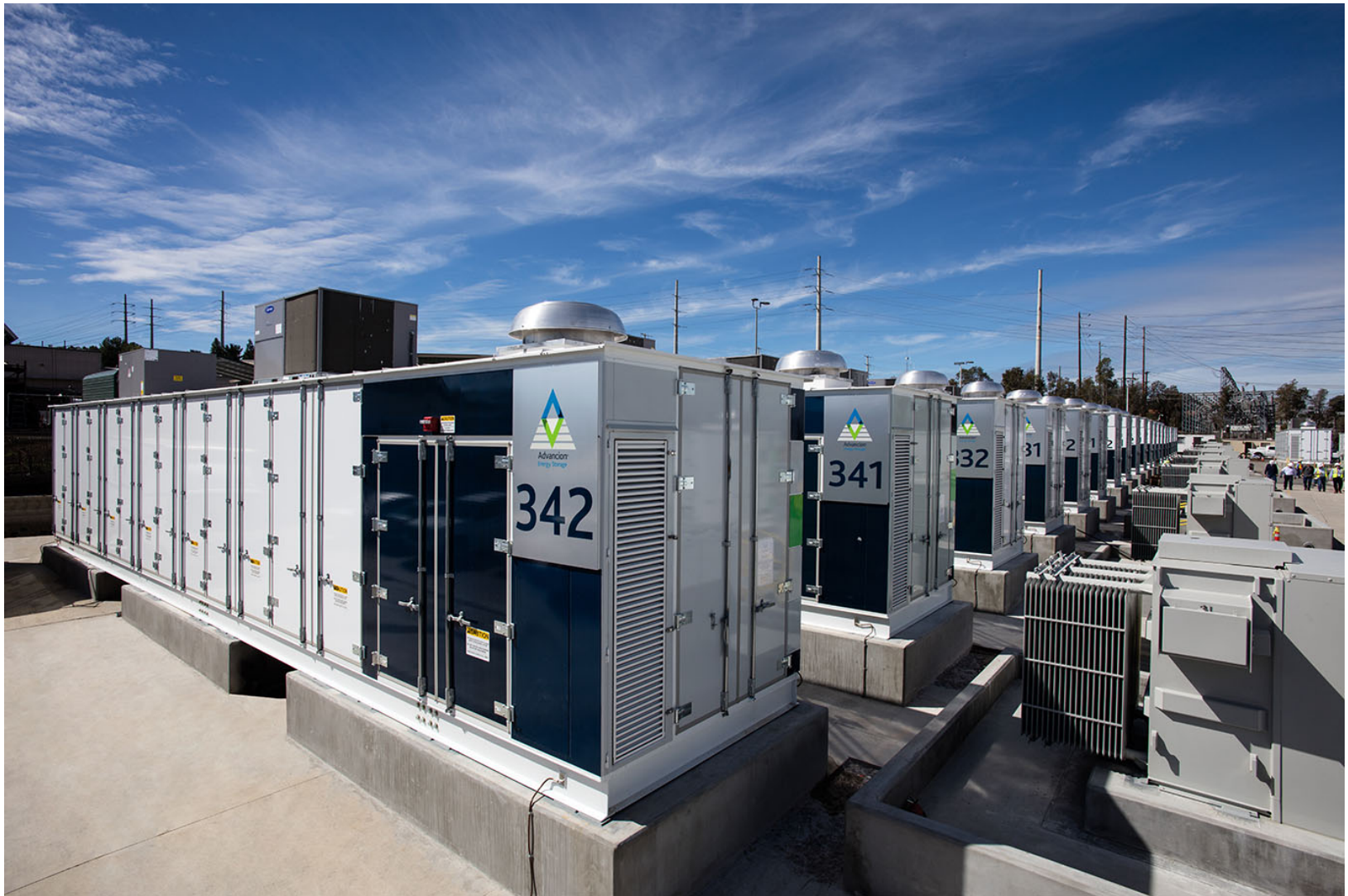
Escondido, California – 37,5Mw lithium ion battery-based energy storage installation
